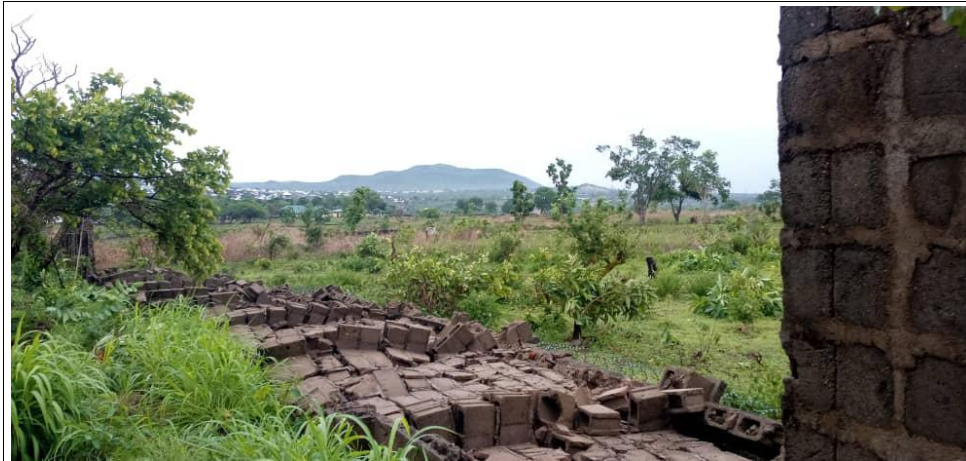
Destroyed security wall
