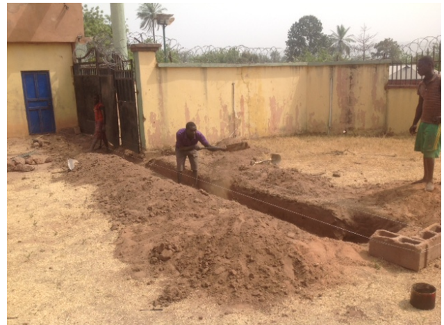
We are digging a trench for a more secure gate at our entrance.
